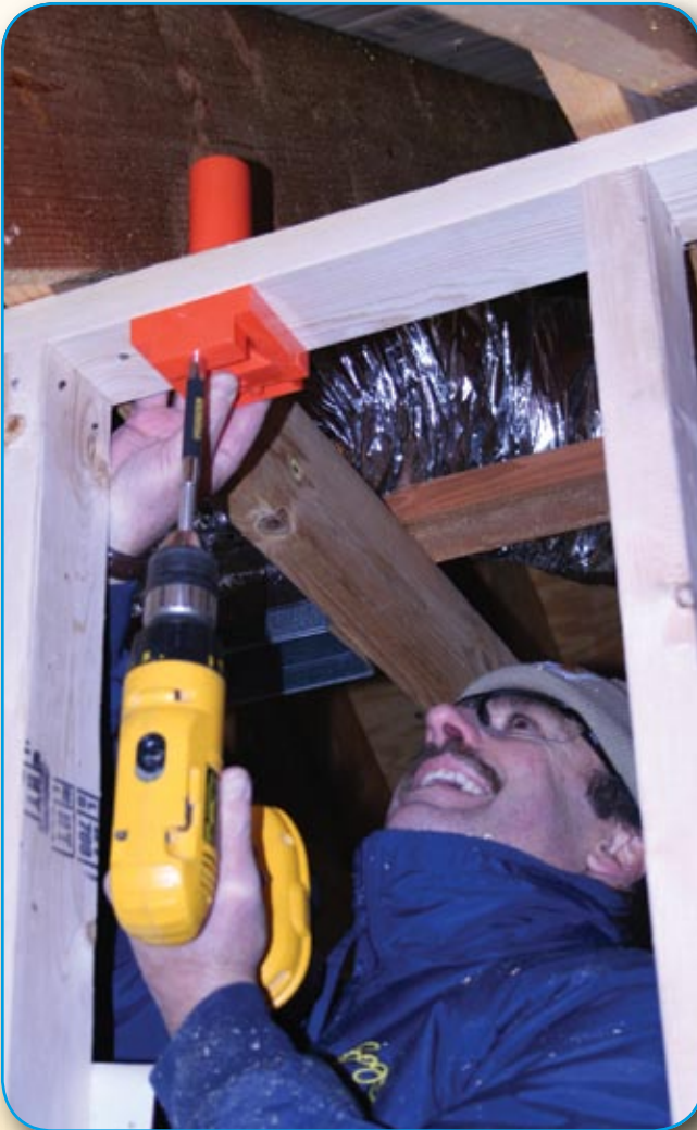
Cable pathways can be placed anywhere in the house, even in the attic.
