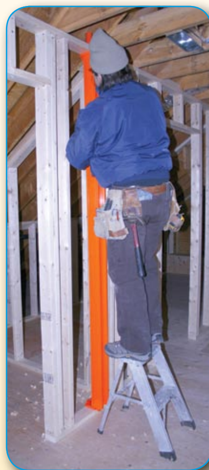
Accessible pathways for cabling are installed before interior walls are closed in.
