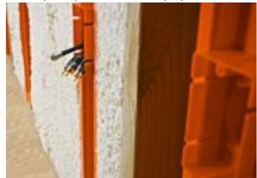
The eXapath system shown in sprayfoam insulation
