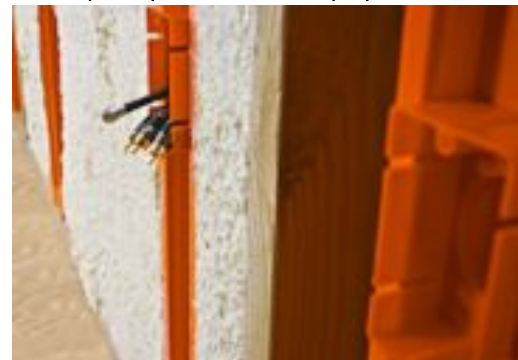
The eXapath system shown in sprayfoam insulation
